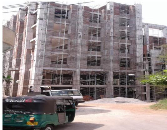
Building complex for the Department of Industrial Management University of Kelaniya - TEC Rs. 500 Mn Physical Progress 48%
