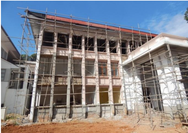
New Building for the Department of Geology Stage 11 - University of Peradeniya - Physical Progress 75% - TEC Rs. 165.8 Mn
