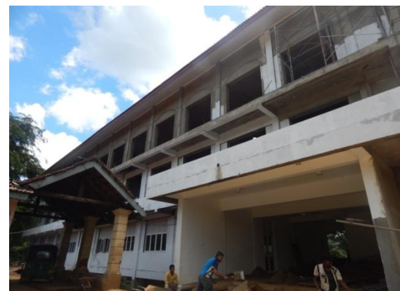
Construction an Administration building with Laboratories and lecture hall for the Faculty of AHS – University of Peradeniya – TEC 157 Mn
